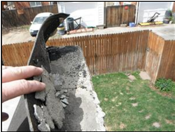
The edges were not sealed properly.
