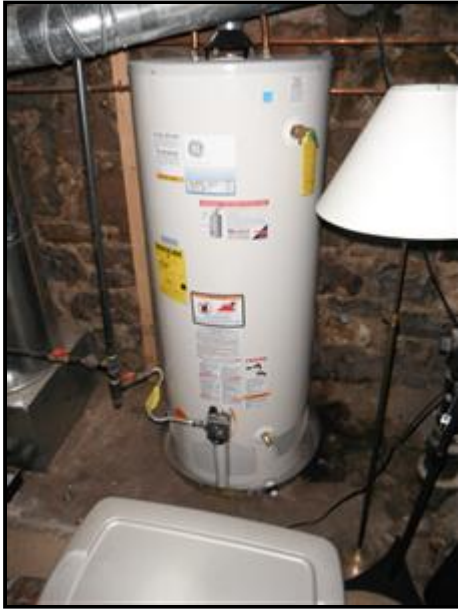
The water heater.
