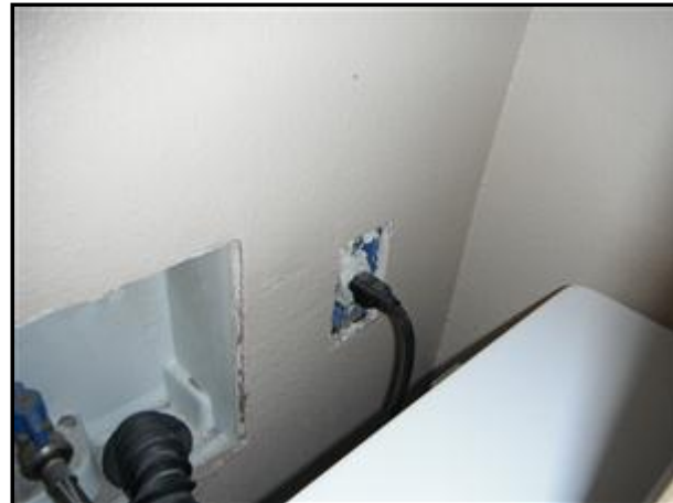
The washing machine junction box should extend to the surface of the wall. It should also have a face plate.
