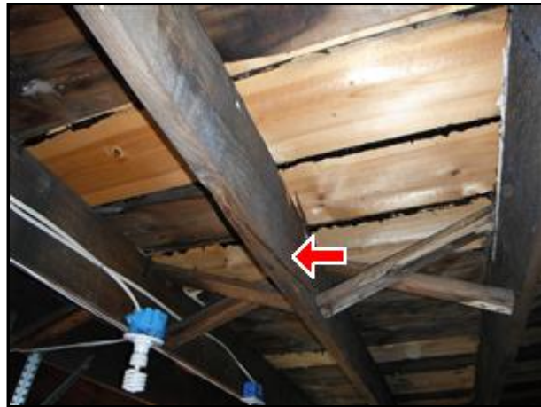
The split joist.
