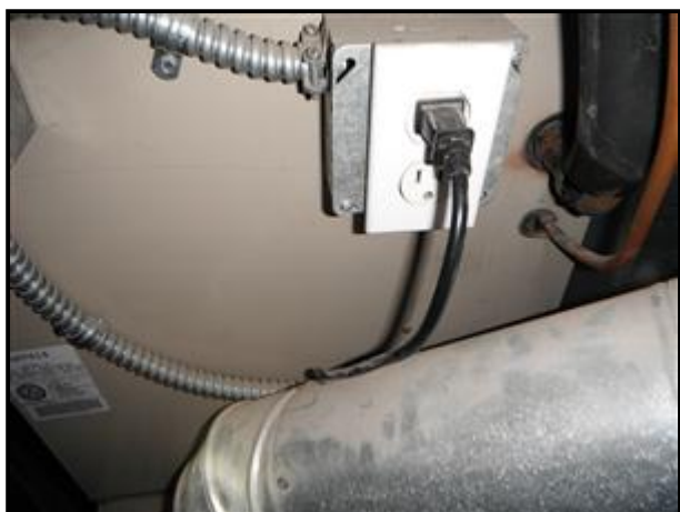
The cord for the condensate pump should not be laying against the furnace vent.
