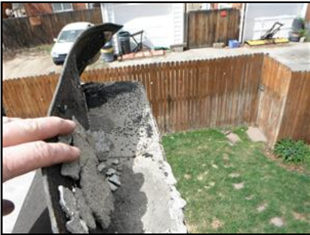
The eadges were not sealed properly.
