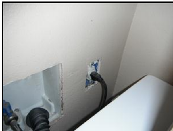
The washing machine junction box should extend to the surface of the wall. It should also have a face plate.
