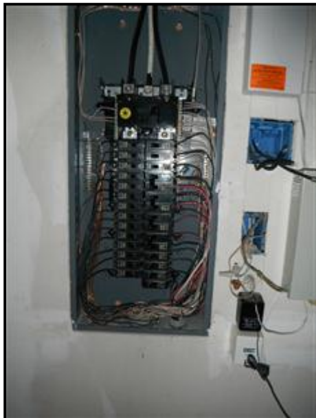
The main electrical panel.
