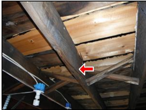
The split joist.
