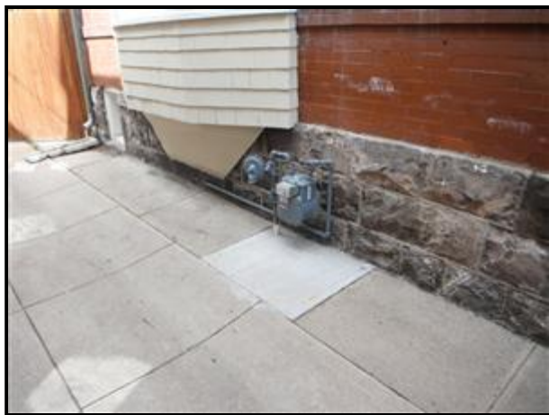
The gas meter.
